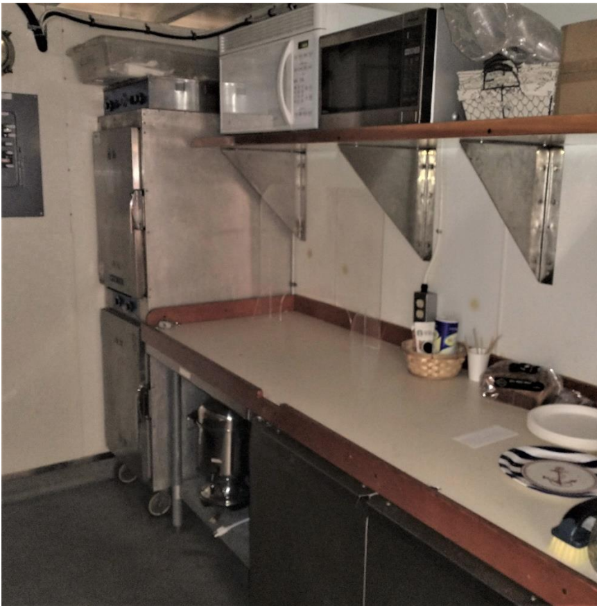
Galley (forward side). Warming ovens, microwaves and a small under counter fridge are shown.
